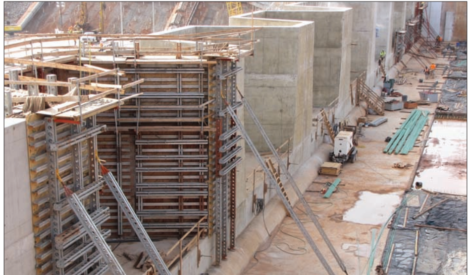
Fuse gates under construction in the auxiliary spillway of Canton Dam, Okla. PHOTOS BY HEIDI WILBARGER
